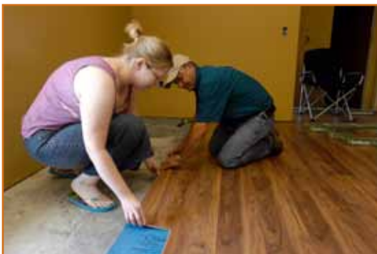
A UHDC self-help family puts in the floor for their new home. Families spend long hours working on their houses contributing as much as 1,500 hours of “sweat equity.” Photo by Karen Segrave.
